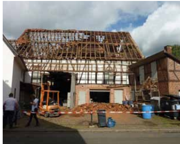
Impact of a tornado in Lumda (Hessen), July 2010
