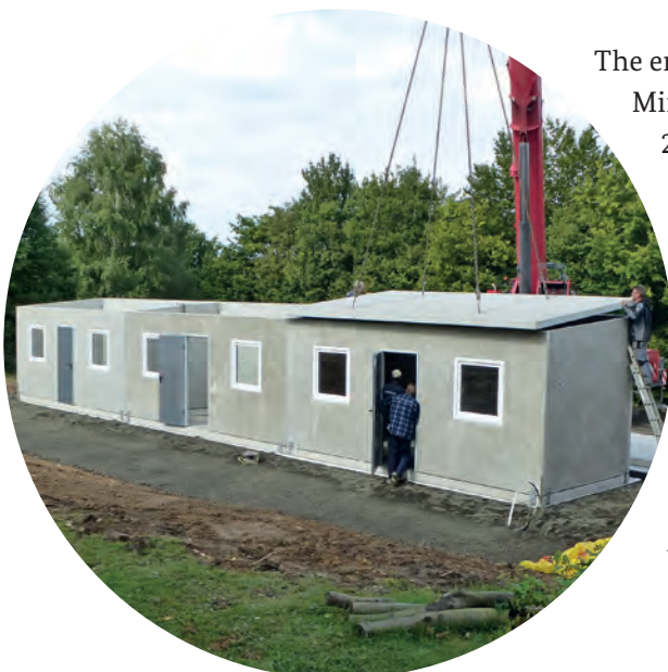
Establishment of initial reception accommodation for refugees at the AKNZ. The sanitary facilities were the most urgent requirement and therefore constructed first.
